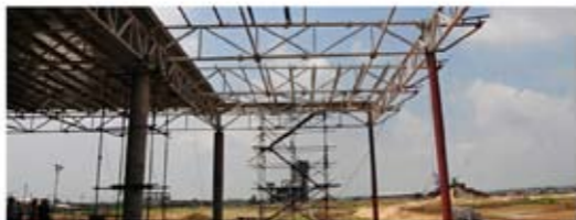
Full swing A file photo of construction work at the Durgapur Aerotropolis at Andal in West Bengal's Bardhaman district. It is due to open this December. A ROY CHOWDHURY
